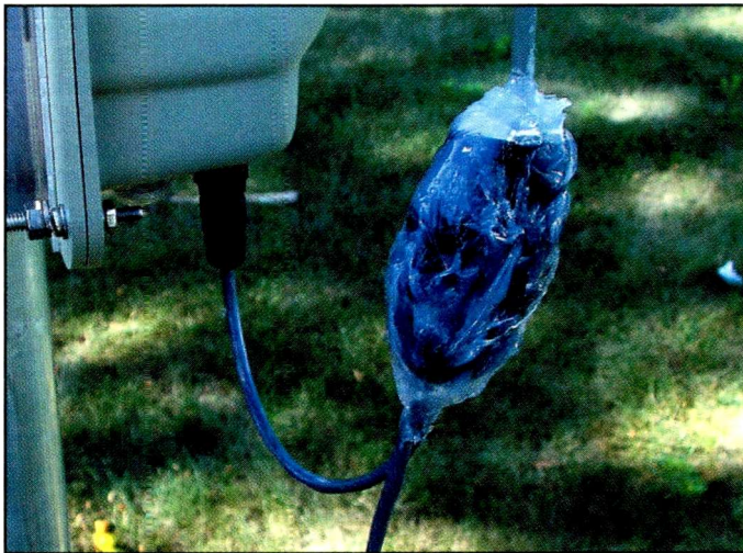
The plug portion of the wiring harness is taped, then covered with silicone sealant (not included) to protect it from the harsh outdoor elements. It's then taped securely to the boom.
